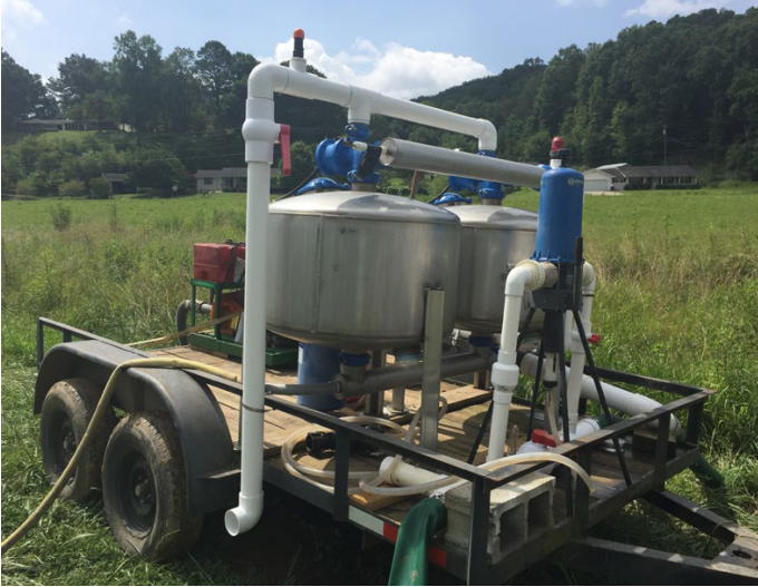
Photo 5: Example of a portable water treatment system used for irrigation.
